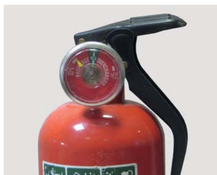
Discharged fire extinguisher gauge
