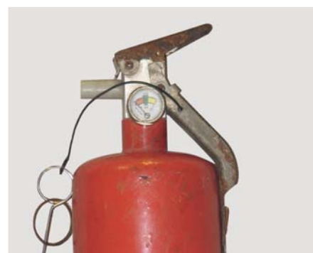
Old fire extinguisher
